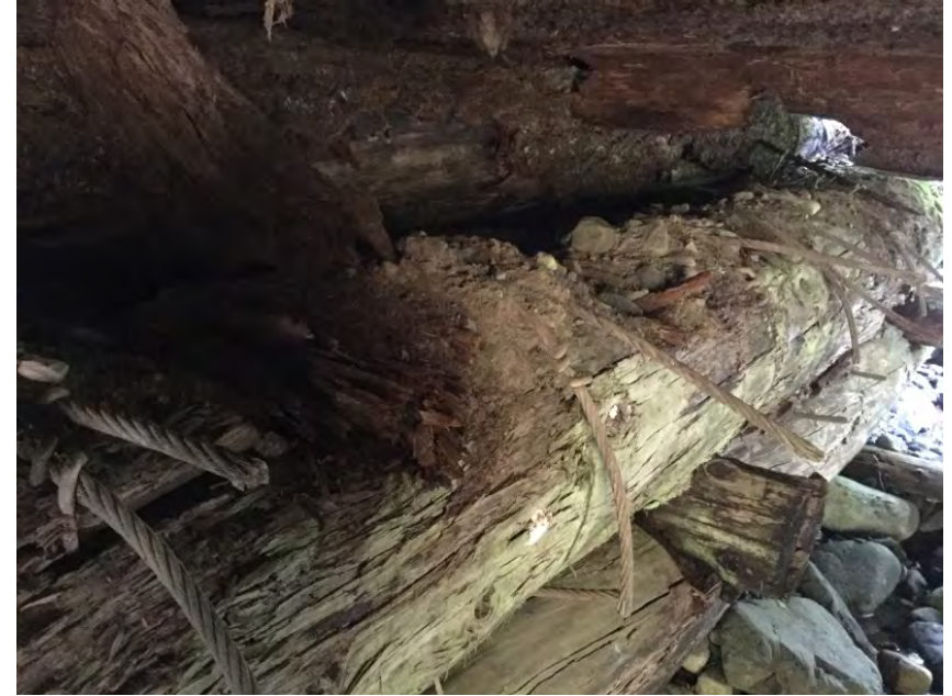
Bearing sill at right bank 1m behind scoured crib
